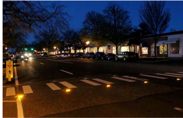
Illustration 1.36: Flashing Crosswalk with 'Yield to Pedestrians' Bollard
