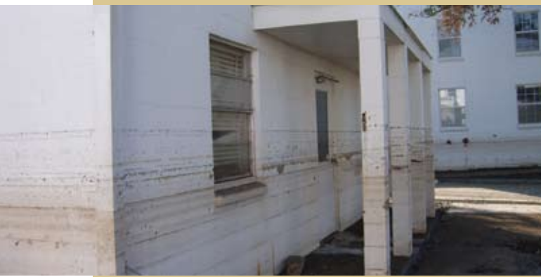
Floodline on exterior of Henson and Williams Halls.
